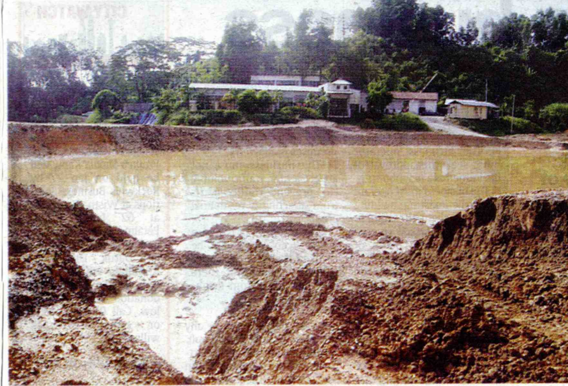
Broken bund: The retention pond does not work as it is supposed to, thanks to a broken bund.
