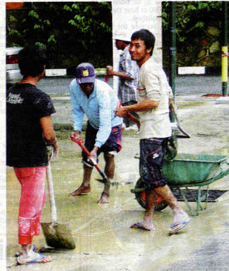
Clean-up crew: Construction workers helping to clear the mud and dirt left behind after the incident.
