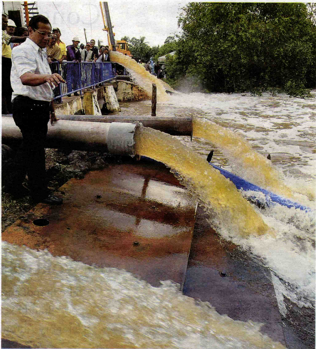
Datuk Ghani Othman inspecting the hydraulic pumps in Senggarang yesterday.
