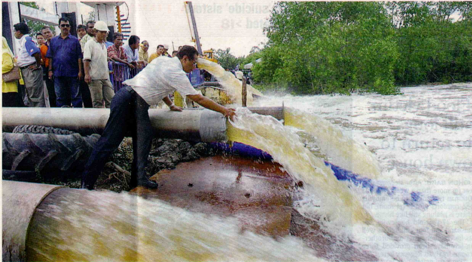
Overseeing ops: Abdul Ghani checking on the pipes used to pump water from Sungai Senggarang into the Straits of Malacca in Johor yesterday.
