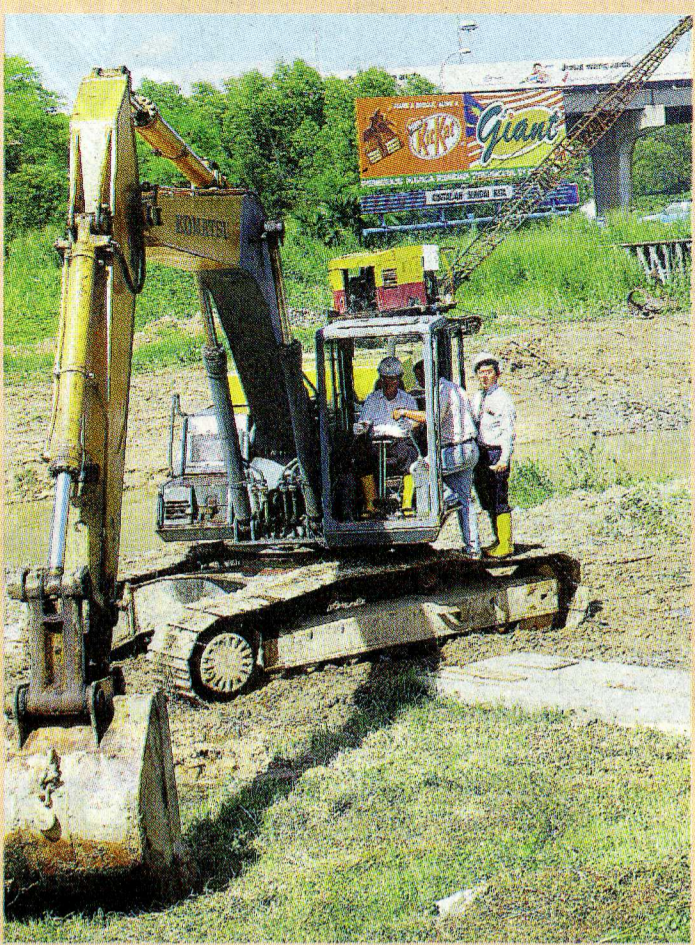
Keizrul in the driver's seat of an excavator at the ground-breaking ceremony for upgrading work at Sungai Damansara and Sungai Kuning in Shah Alam yesterday.
