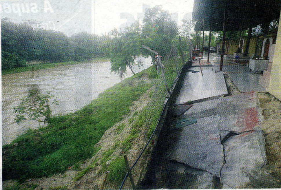
PRECARIOUS SPOT: The Hindu temple in Old Klang Road, near Kuala Lumpur, is in danger of collapsing following soil erosion after a landslide caused by heavy rains.
