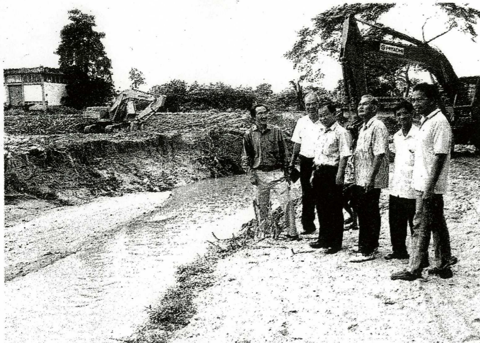
Yap (far left) and Taman Selamat residents looking at the progress of bank strengthening works along Sungai Merbau.
