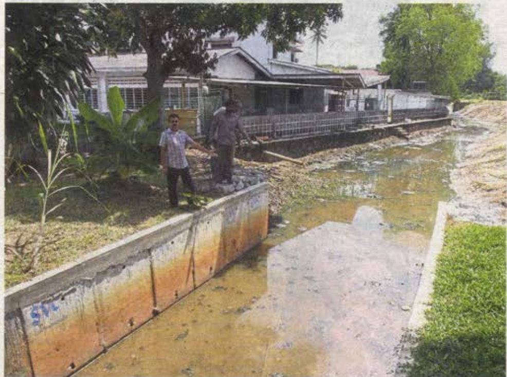
Ravinder (second from left) and members of the Sikh community showing the uncompleted monsoon drain. Work on the project stopped last November. — UU BAN/The Star
