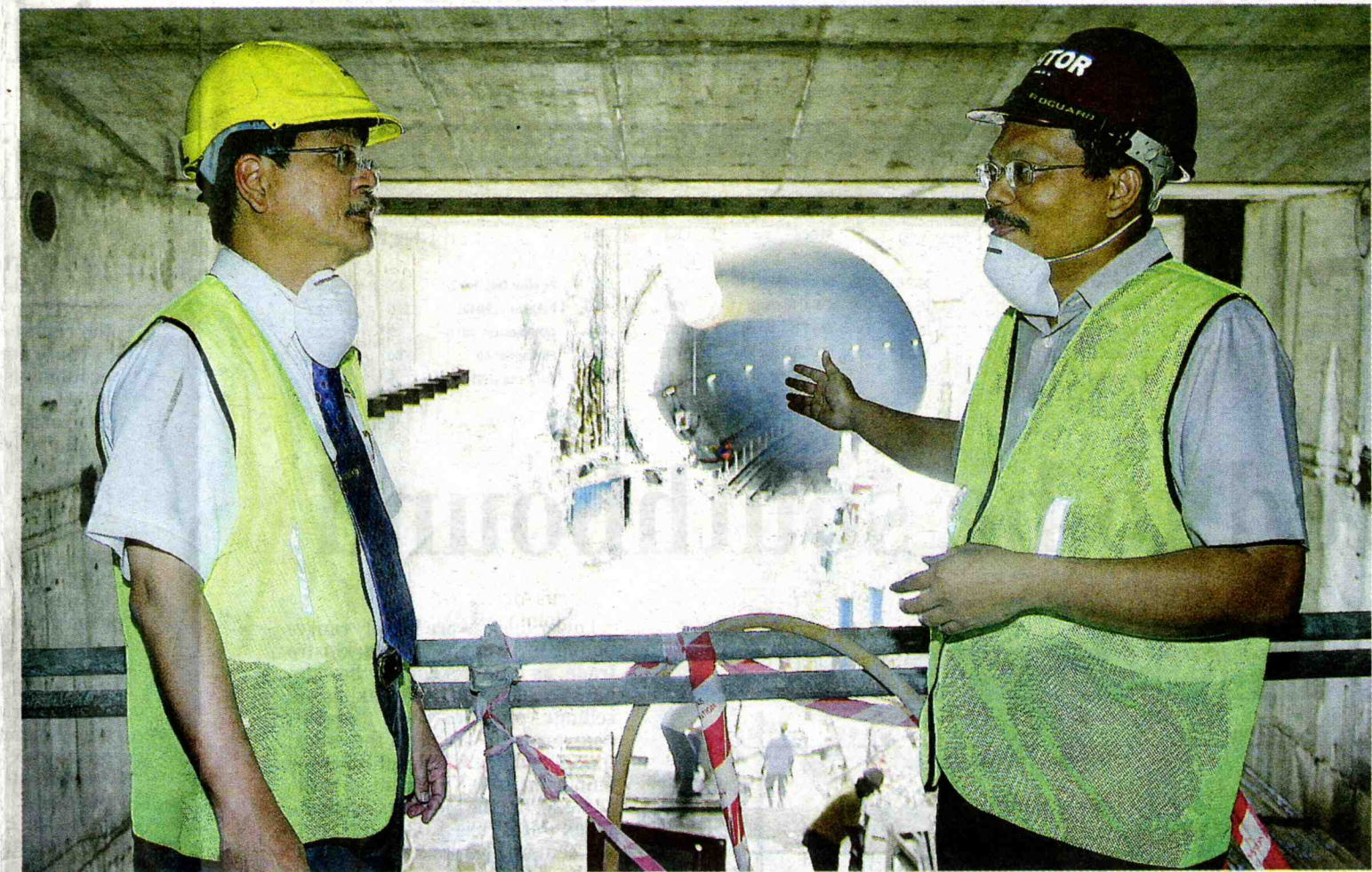
Azmi (left) briefing Keizrul on the progress of the dual-purpose tunnel. The project is expected to be the long-awaited solution to massive flooding and traffic woes on the key Sungei Besi roadway leading into the city centre.
