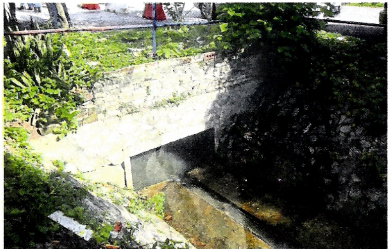
The small drain and waste trap slows down water flow and results in an overflow which then floods nearby houses.
