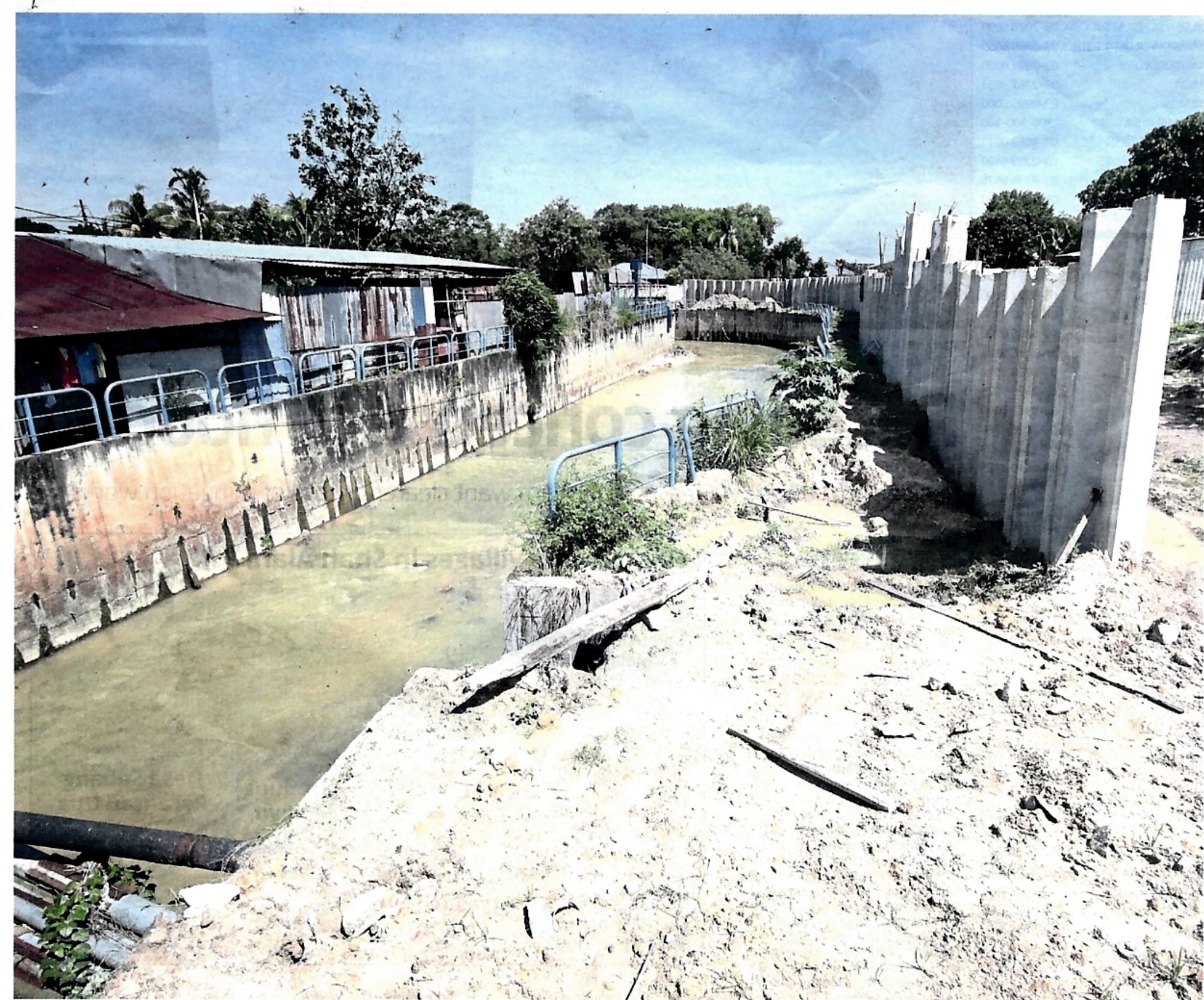
Preventive measures: The mitigation project includes setting up retaining walls and dredging works along a 2.1km stretch of the Sungai Pelempas where the floods have occurred. — SADIQ SANI/The Star
