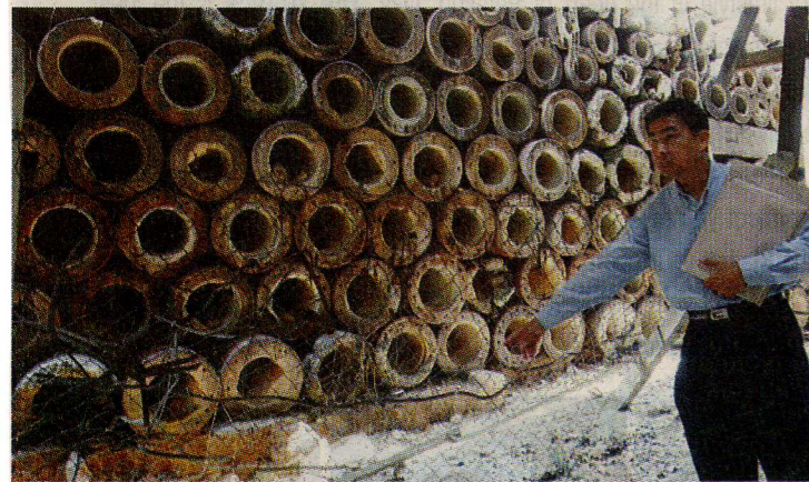
Yee checking on the factory's fence which has collapsed due to the construction work.
