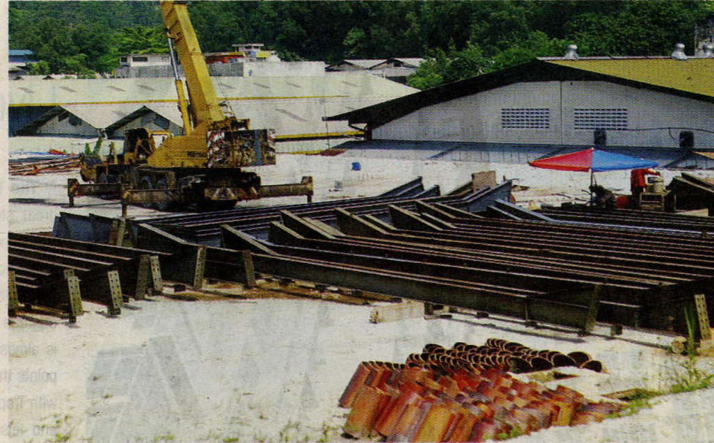
Work still being carried out on the project despite a stop work order by MPS.
