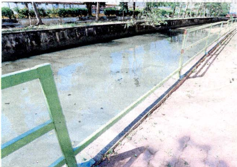
The missing safety railing along Sungai Raja in Alor Star. PIC BY AMRAN HAMID
